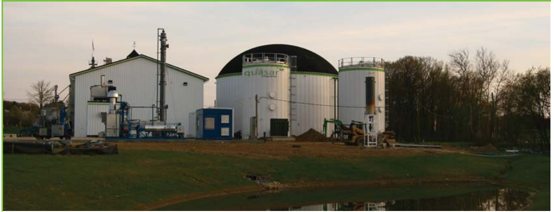
quasar's F550 system on the OARDC campus
